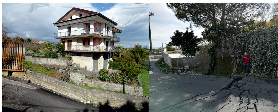
Fig. 2 - Earthquake surface rupture across the road (right) and a house (left) located a few meters apart in the vicinity of Santa Maria La Stella; notably, the main rupture is located approximately in the middle of a scarp which is the long-term morphological expression of the fault, already censored and mapped with great detail in the Ithaca Database of ISPRA, available since 20 years ago. In spite of this knowledge, the house, built right on the fault trace, was restored and licensed to be widened just before the event. Following the December 26, 2018, earthquake, the house is no longer habitable, being crossed by severe fractures and slightly tilted.
