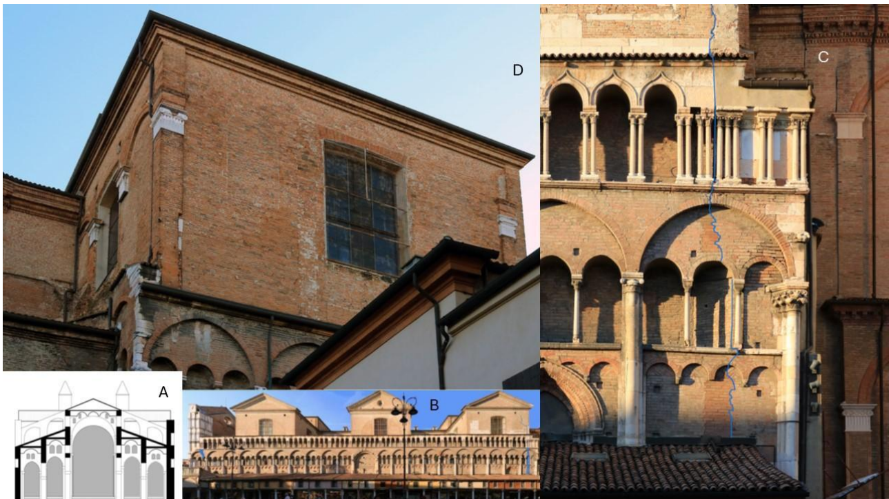
Fig. 1 – A reconstructive cross section of the Ferrara Cathedral after the 13 th century post-seismic restoration (drawing by A. Toma and V. Vona), B southern side of the Cathedral, with the main structural lesions induced by foundation settlement and seismic acceleration depicted in blue, C the south-eastern corner, with post-seismic collapse transept reconstruction in a backward position and “wall sewing up restoration” by reddish bricks, D the Renaissance transept rebuilt at the end of the 15 th century and partially collapsed during the earthquake of 17 Novembre 1570.
